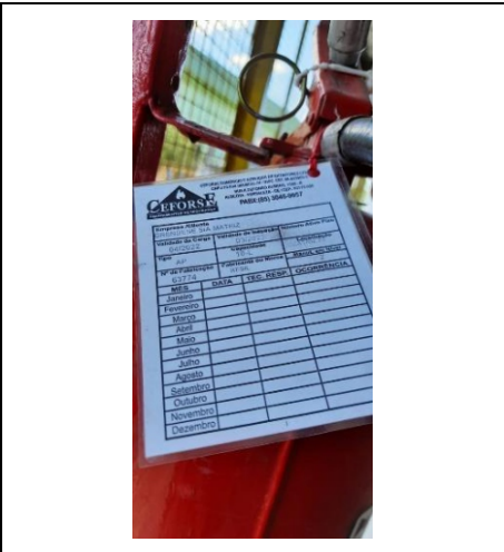
NC: fire extinguisher
